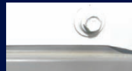
Minimal corrosion is detected along cut end of panel with Edge-Rust Inhibitor application.
